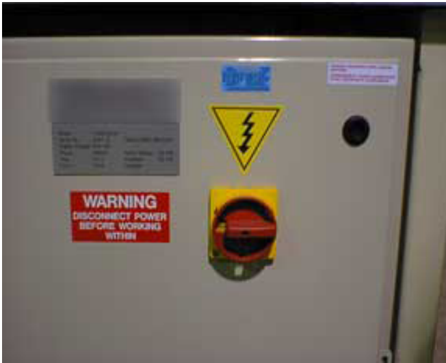
Photo 5 – Disconnect with E-Stop Colours indicates that this device is intended to be used for EMERGENCY SWITCHING OFF.
