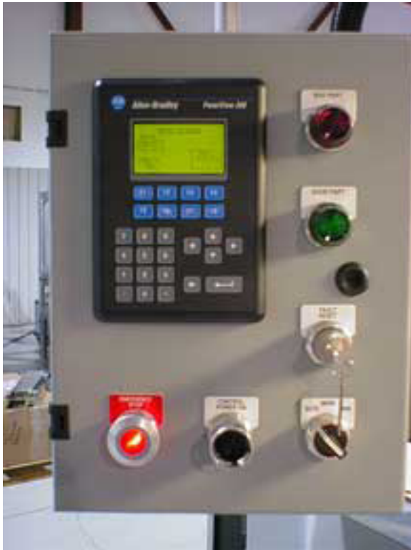
Photo 3 – This more modern button is non-compliant due to the RED background.
