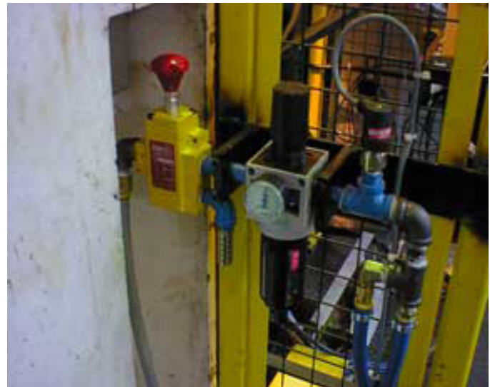
Photo 6 – Pneumatic E-Stop/Isolation device (on left)
