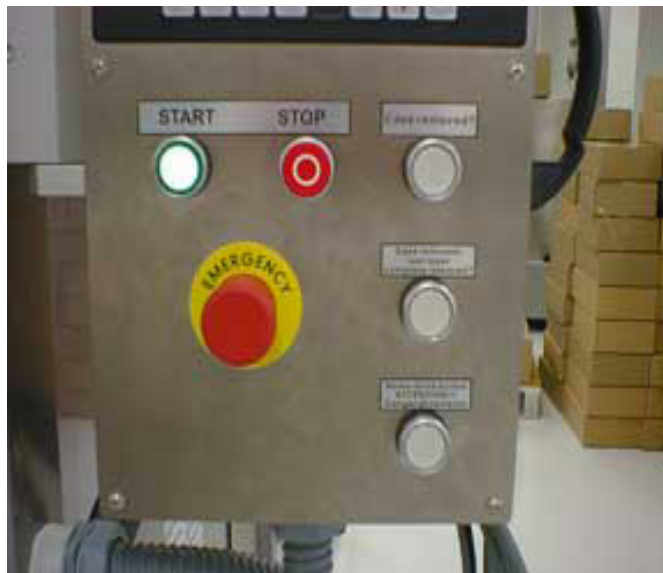
Photo 4 – This E-Stop button is CORRECT. Note the Push-Pull-Twist operator and the YELLOW background.
