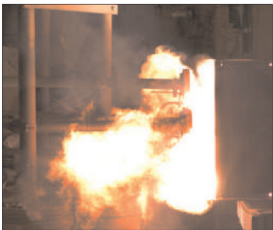
Figure 1 – An example of an arcing fault [1].
