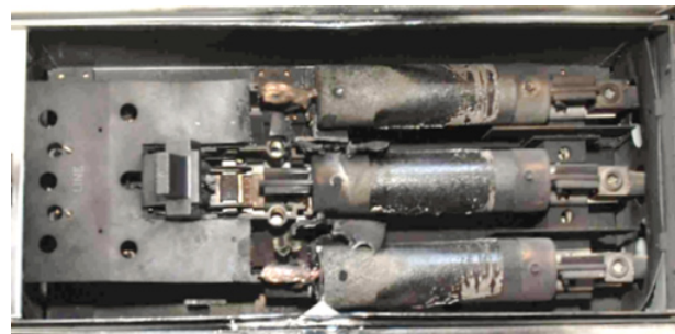
Figure 5 – Arc damage to the terminals of the mechanical disconnect and the fuses.
