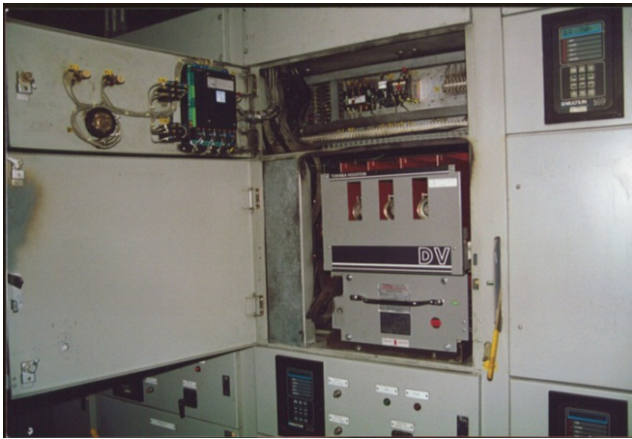
Figure 4 – 5.0 kV, 400 A replacement circuit breaker at the power plant.
