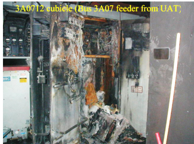
Figure 2 – High Energy Arcing Fault (HEAF) at Diablo Canyon Power Plant [2].
