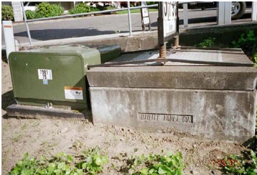
Figure 1: Restored transformer site picture
